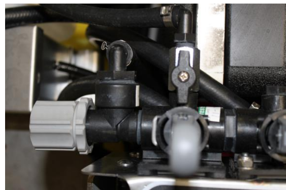
(Hose reel Chrome Valve in open position)
