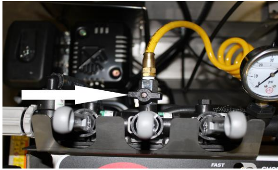
(Hose reel Chrome Valve in closed position)
